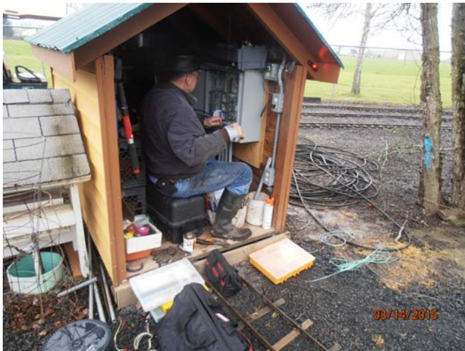
Alan installs signal controllers at the south end of the garden. (...a very wet and rainy day...)
