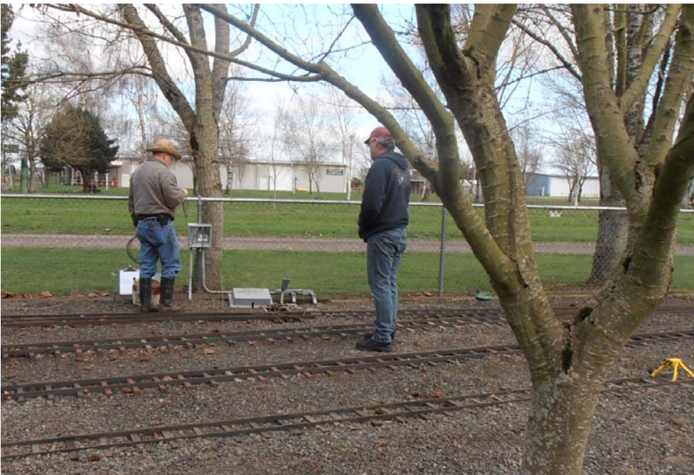
New control box.
