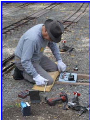
...Paul is getting ready to test the electrical turnout system...
