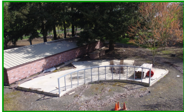
Phil L., Vern & Ernie installed roundhouse door frames Roundhouse Door Frames Placed February
