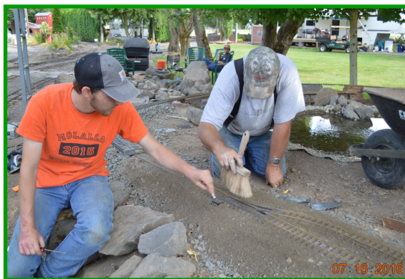
Bryson & Ernie ballast the G-scale tracks. Coyote Ridge G-Scale Railroad, Ponds & Stream July
