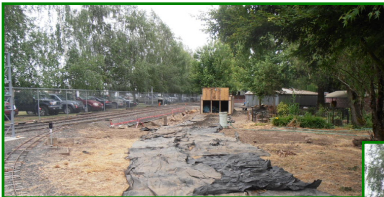
Saturday July 1 st : Work was started on placing track to car barn. Geo-fabric was put down and placing gravel base was started.
