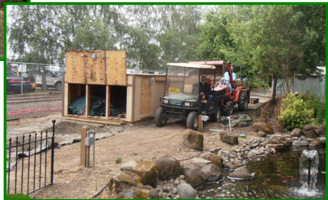
The Easy-Go and Terry's tractor were used to move gravel for the new track alignment.
