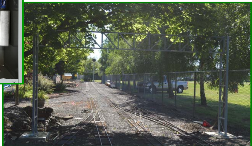
Showing location of signal bridge that will indicate position of switches for Double Crossover
