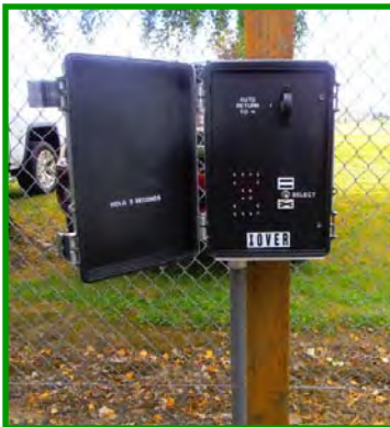
The cabinet to control the positions of the cross-over switches is located on a post on the south side of the tracks in advance of the signal bridge.
