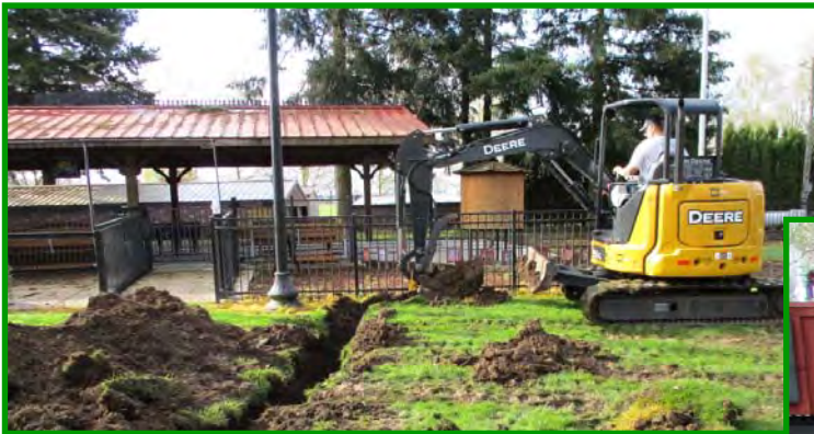
Evan operates the excavator. The trench is being dug to allow Willow Creek to tie into Powerland's improved water system.
