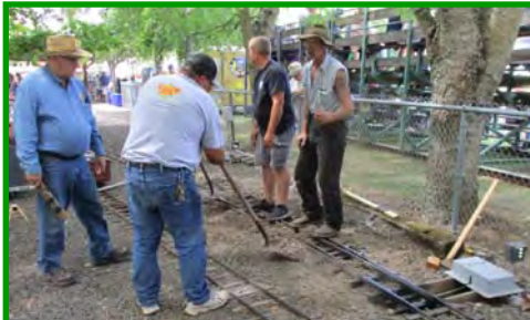
Tree roots disrupt a switch at the station entry track. The train gang makes an emergency repair. Note how the tie along the fence has been raised by the root.
