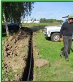
The new 2-inch water line has been extended to just east of the Vits Crossing where it will be connected to the existing WCRR system.
