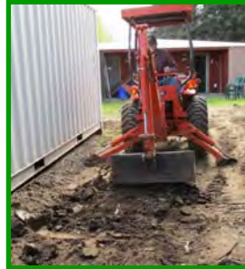
Steve uses his backhoe to grade the area and expose remaining roots.
