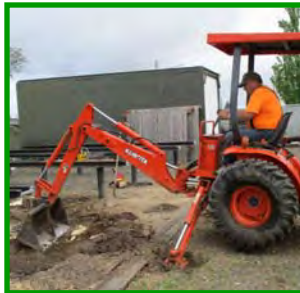
Ernie removes remaining poplar tree roots that the stump chipper could not reach.
