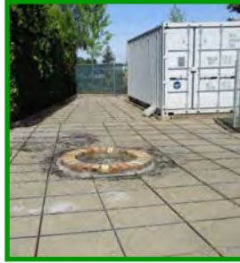
Forms and reinforcing steel are in place for the new slab. The fire ring has been moved slightly to the south and west. The firebricks surrounding the new ring location were formerly used as the liner for SP&S 700 firebox.
