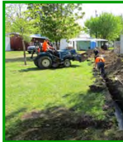
Bryson, Dave and Ernie place round gravel drain rock above the waterline prior to backfilling the trench. This french drain will help disperse rainfall drainage from the new ICP slab.
