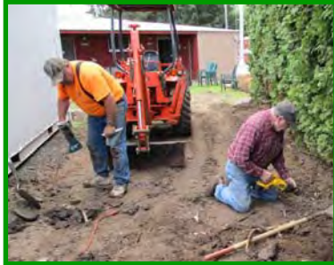
Ernie and Steve Scharer cut remaining tree roots in preparation for the proposed slab.
