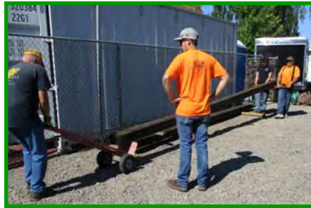
Bridge timbers donated by the Trolley Museum are moved to the platform.
