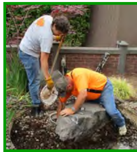
Jesse and Ernie remove roots from the memorial garden bubbler pool. Roots from the poplar tree had filled the pool. Excess round rock was moved to the ICP landscaping area.
