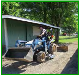
Mark grades the gravel placed between the ICP and the building to the north. The gravel provides an all weather walking surface. It extends from the front of the buildings westward to the end of the fenced area.
