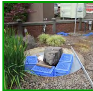
Old milk crates were cut and installed to reduce the amount of round gravel required to fill the pool and increase the volume of stored water.
