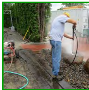
Dave power washes the ICP boulders and the round gravel that was salvaged from the Memorial Garden bubbler pool.
