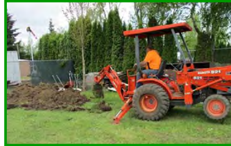
Ernie continues excavating the waterline trench to the west. This will allow a tie to the existing water system and provide two new all weather hose bibs outside the fenced area.
