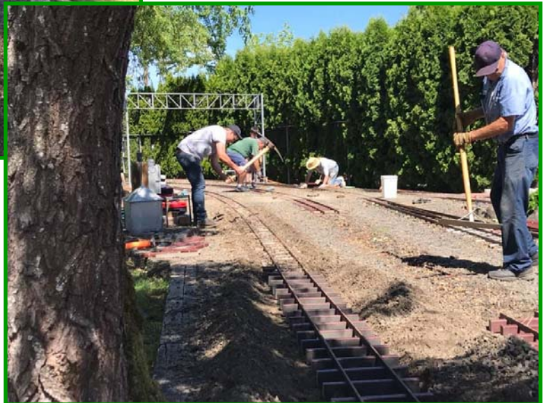
The crew replace the track panels with the new Trex ties installed.
