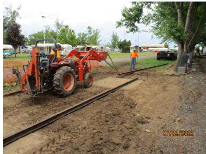
The Trolley Museum donated rails to support the caboose. Here they are being dragged into place.
